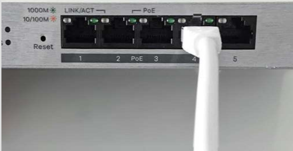
Figure 3: PoE Port of Switch, connected with Beacon
