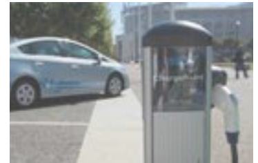
EV Charging Stations
