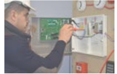
Fire Safety Alert Systems
