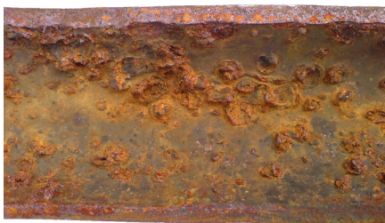
MIC Corrosion Inside Pipe
