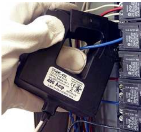
Photo 2: Install CT Around Conductor.
