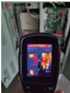
Detecting of Power Distribution Cabinet
