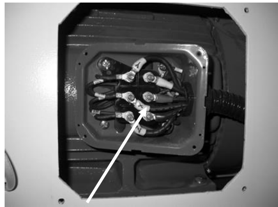
Motor electrical terminations (cover plate removed)
