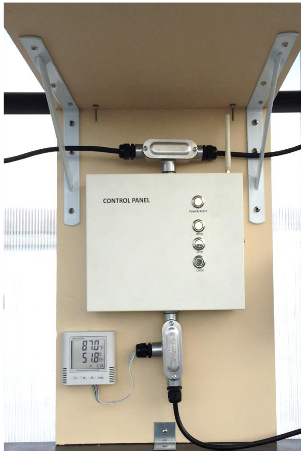
Typical wired control panel setup
