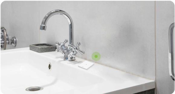
Bathroom (Toilet sinks, washing machine)
